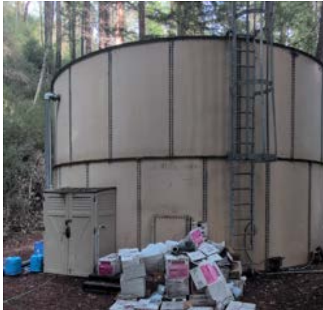
Figure 2-3: Well No. 4 Tank (Inlet Piping Shown)
