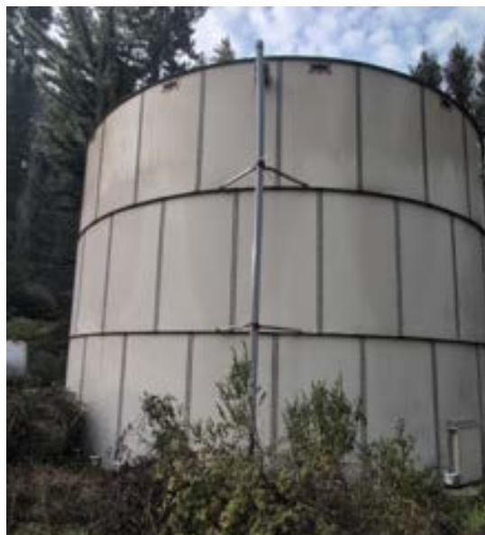
Figure 2-2: Jamison Tank Bolted Steel (Inlet Pipe Shown)
