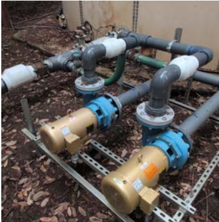
Figure 5-2. Tank #4 Booster Pump Piping
