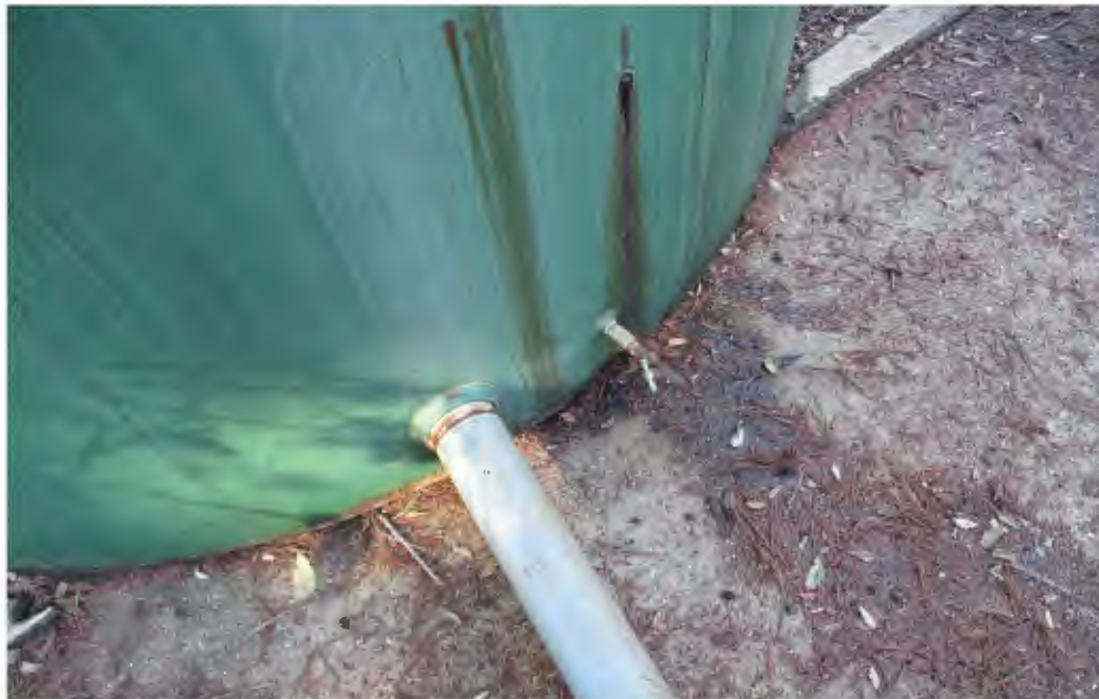
Corrosion and Leaks in the Tank Sidewall
