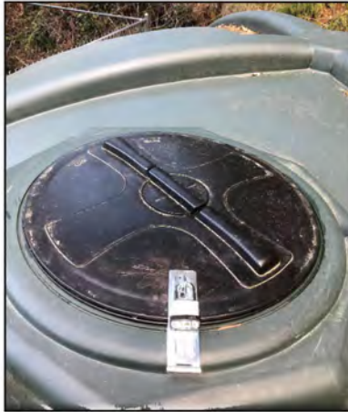
Figure 10: Roof lock on China Grade Tank.
