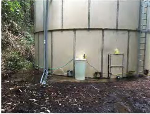
Figure 1. Temporary Disinfectant Injection Configuration at Well # 4
