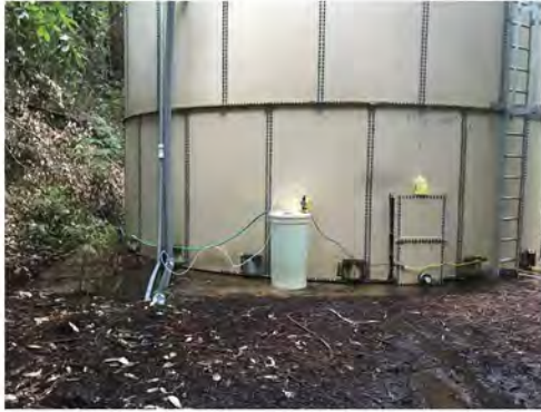
Figure 1. Temporary Disinfectant Injection Configuration at Well # 4
