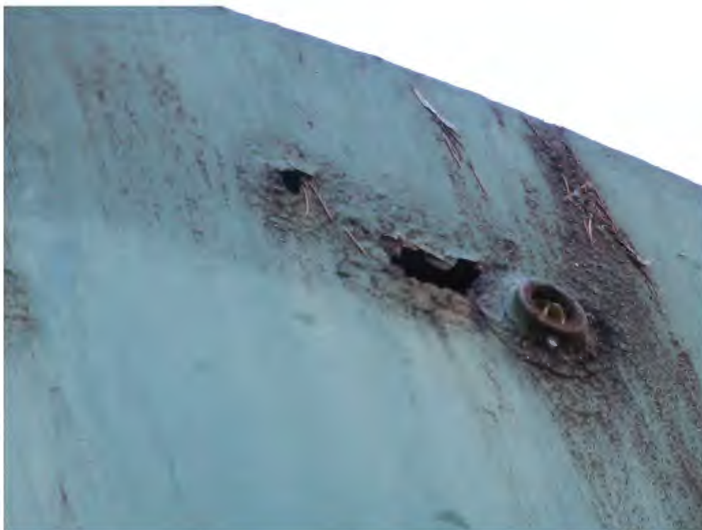
Enlarged Image of Tank Sidewall Holes
